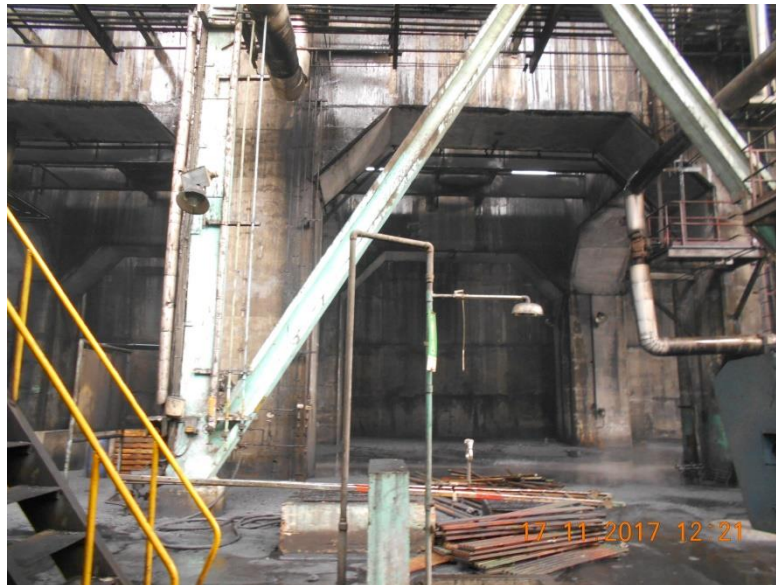
Safety shower location
