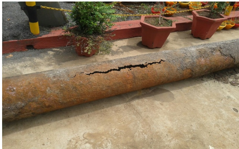
A VIEW OF SEVERELY CORRODED PIPE
