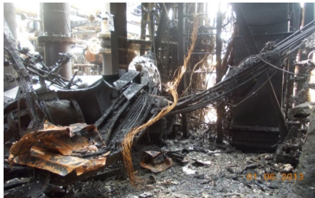
Burnt Instrument & Electrical cables
