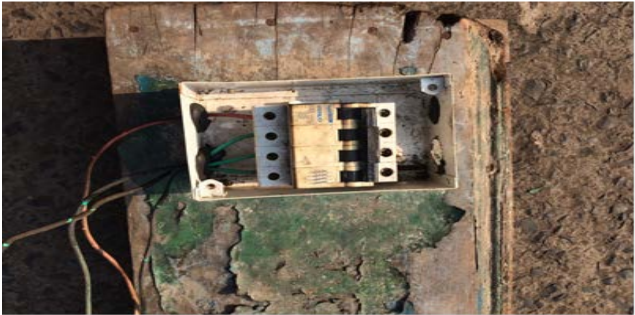
Non FLP switch Board –source of Ignition
